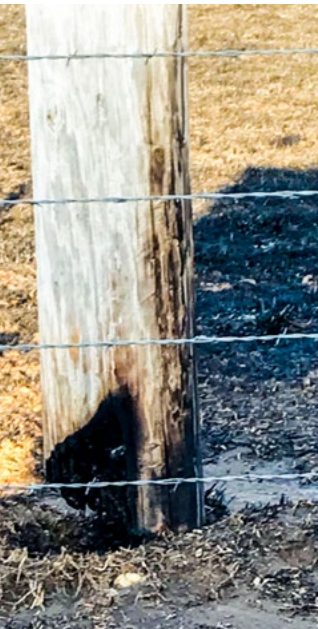
Make safety a priority and take special considerations when burning near electric utility lines.
